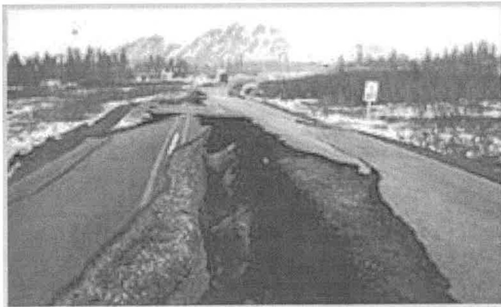
Photograph of cracked road after earthquake
